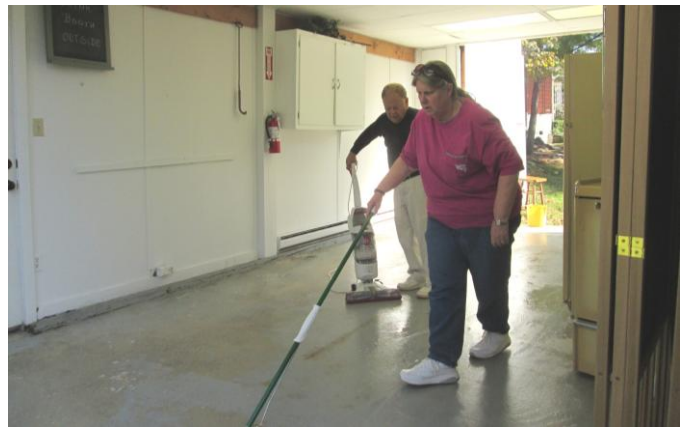
Lou and Kathy Trent cleaning the floor of the Annex in preparation for painting, October 22, 2015.
