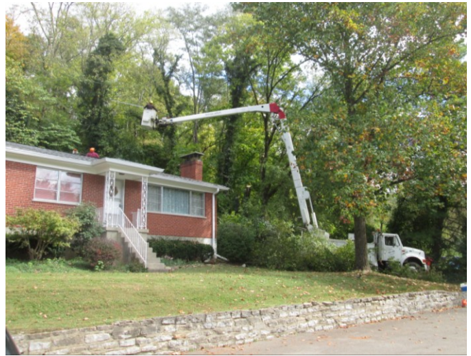
The Dave Vogel Landscape Company trimmed the trees overhanging the Brick House in October 2016.
