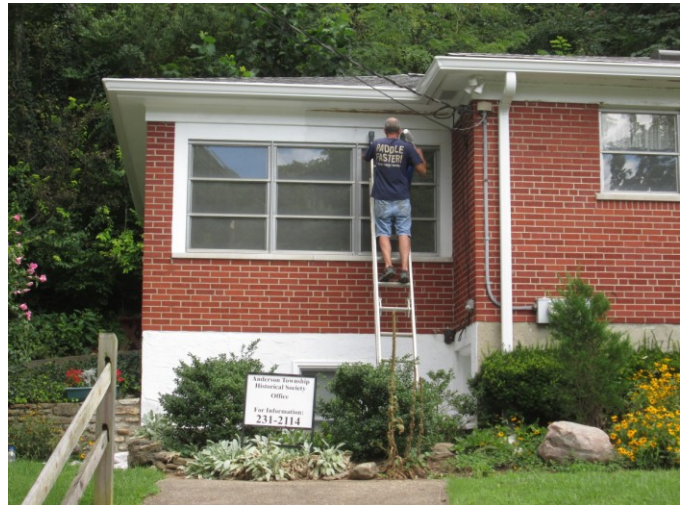
Mike Bottom scraped and painted the wood trim on the Brick House along the south side of the house.
