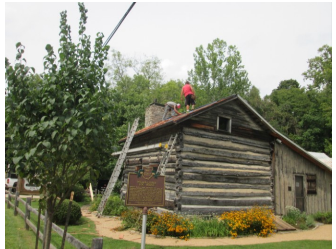
A new cedar roof was installed on the front roof of the historic ATHS Miller-Leuser Log House by Brandstetter's Kanga Roof in August 2018.
