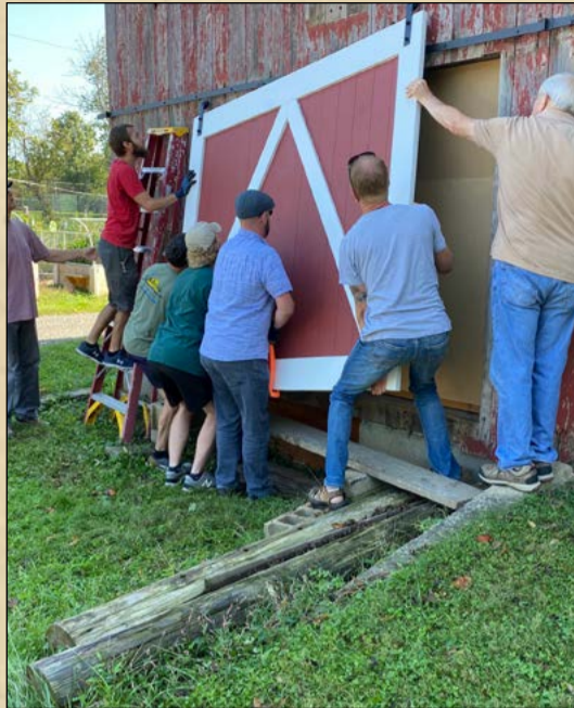
The first new barn door is hung on a new track. Former President Don Perry has designed and built the doors and our volunteers brought their strength to the moment!
